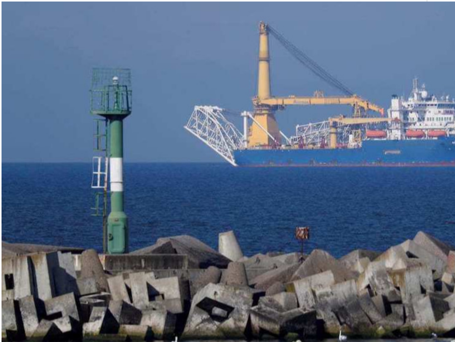
Construction of the Nord Stream 2 gas pipeline, near the Baltic Sea port of Baltiysk, Kaliningrad. (Photo: Reuters)
